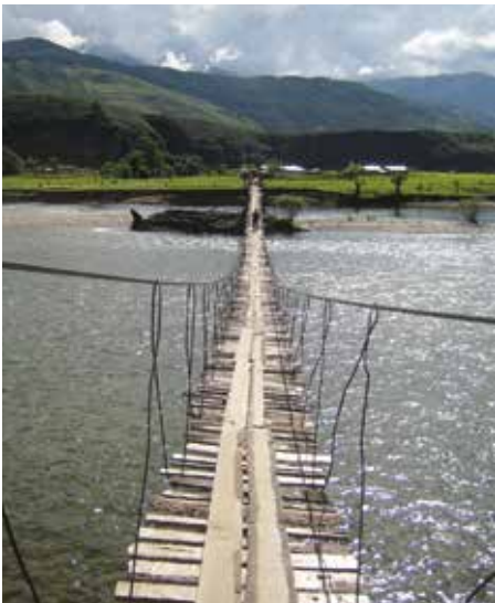
Fig. 11: Suspension bridge over the Siyom River, Mechuka Valley. Photo by Hartwig Schepker.
