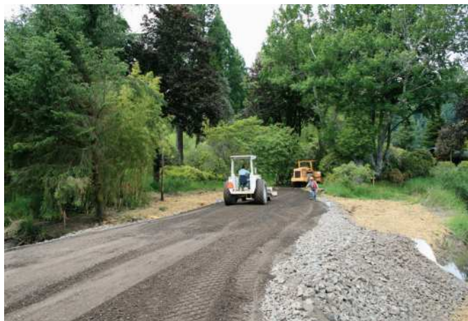
New access road to main garden nearing completion. Photo by Gordon Wylie.
